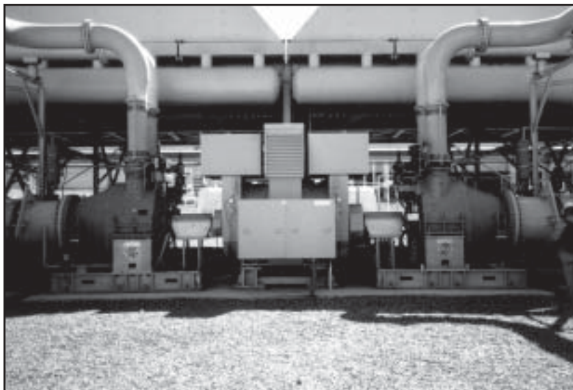
Brady Power Plant new 5-MW binary generation unit showing the generator in center and 2 turbine power units, one on each side of the generator. Photo by R. Hess, 2002.
